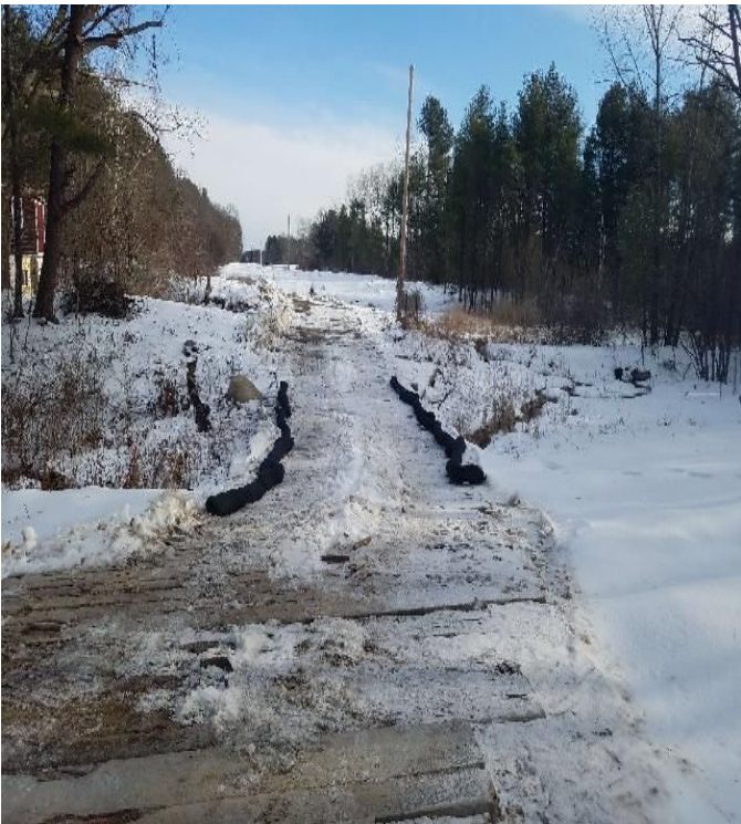
Fig 11: Filter sock installed on timber-bridge over stream NS8, between Strs. 102 and 103. Viewing northeast. (01-06-20).
