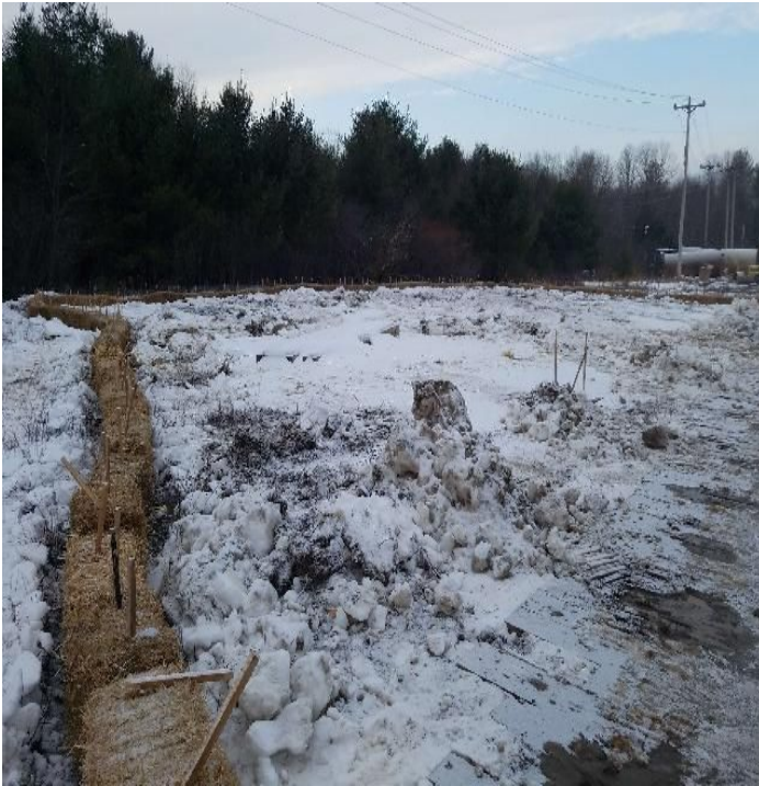
Fig 17: Crew finished installing straw bales around perimeter of turtle nesting area. Viewing southwest. (1-08-20).
