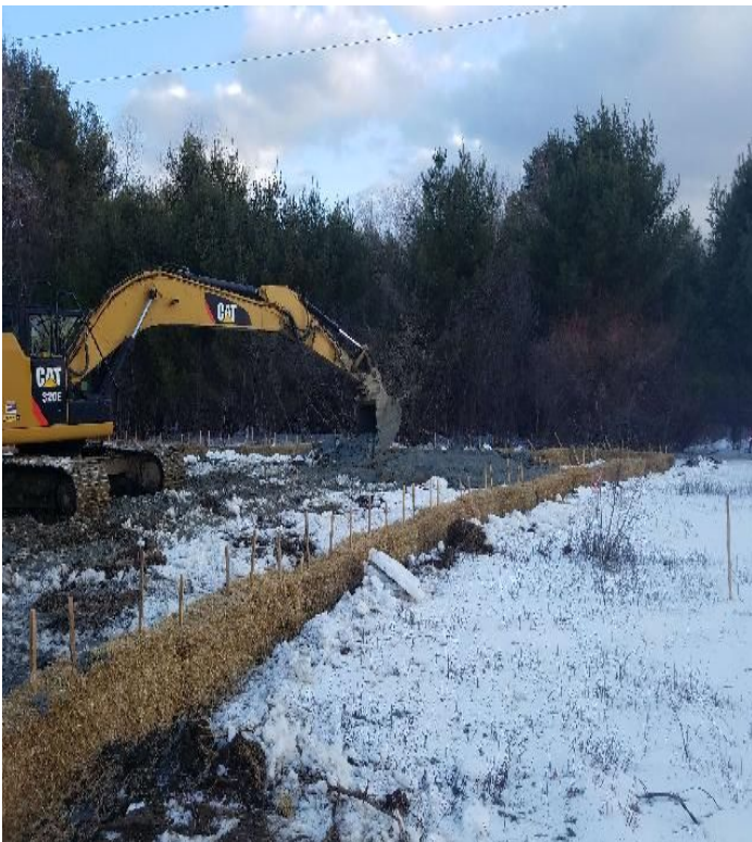
Fig 19: Crew spreading soils to build up designated turtle nesting area. Viewing south. (01-08-20).
