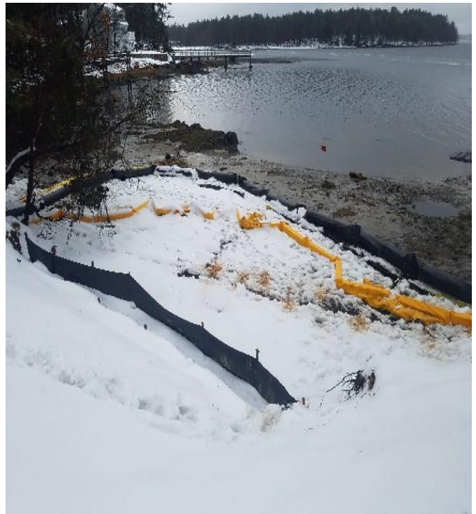
Fig 4: BMPs and turbidity curtain at Gundalow landing/east side of the Bay. Viewing south. (01-02-20).
