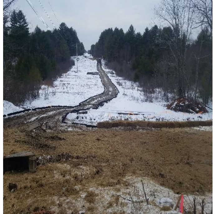
Fig 6: Crew finished installing BMPs on access through wetland DW31 and prepped the site to begin excavation for Str. 57 foundation. Viewing west. (01-02-20).
