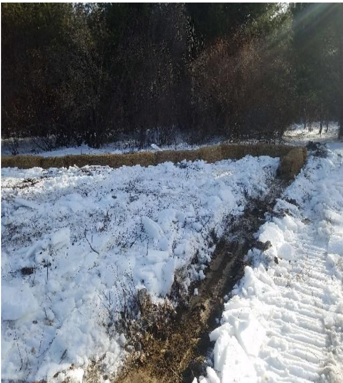
Fig 15: Crew installing perimeter sediment controls for soil spoils from Str.48. Designated turtle nesting area. Viewing east. (01-07-20).
