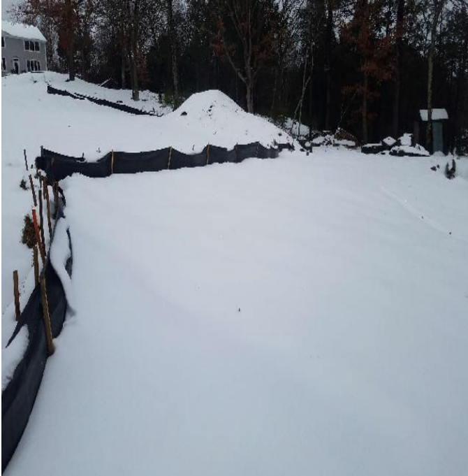
Fig 1: Silt fence installed on slope at Getchell property/west side of the Bay. Viewing north. (01-02-20).
