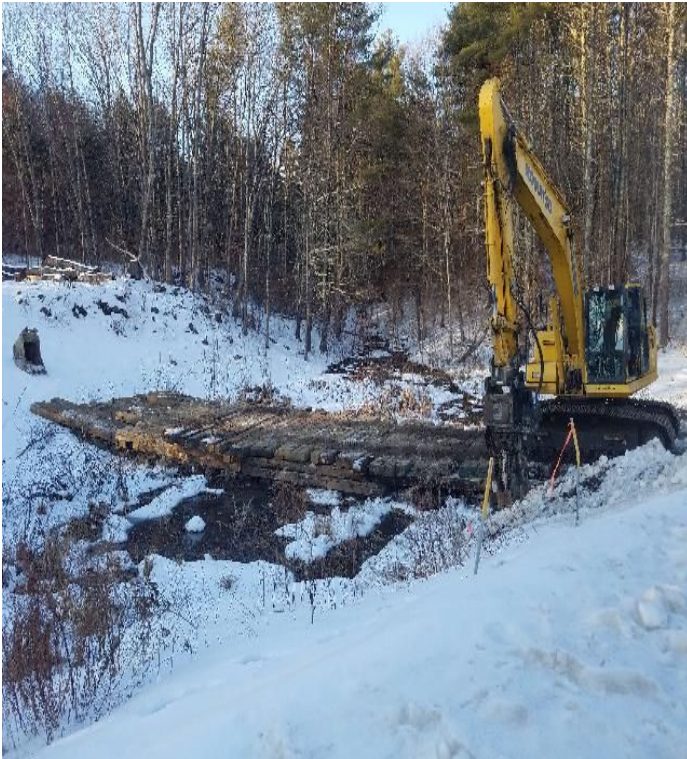
Fig 21: Crew building timber bridge over wetland DW29, off of route 108. Viewing west. (01-08-20).
