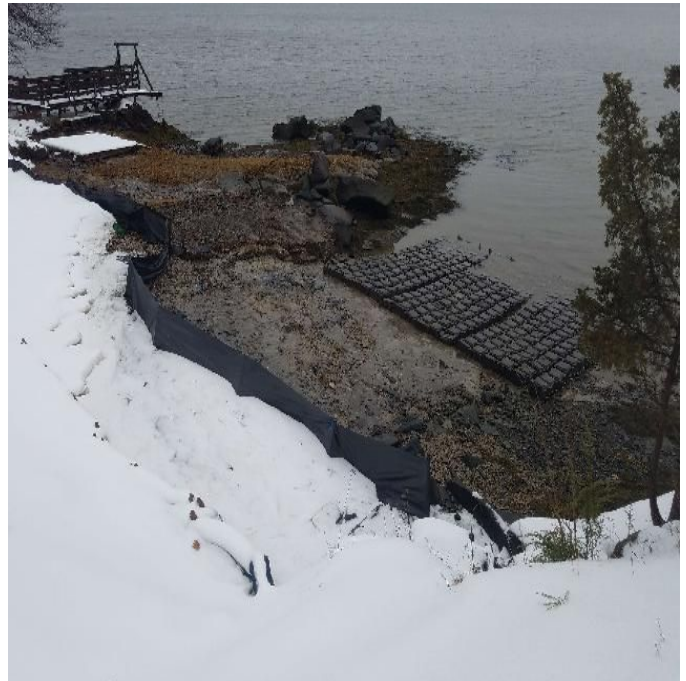
Fig 2: BMPs and concrete mattresses at Getchell property/west side of the Bay. Viewing north. (01-02-20).
