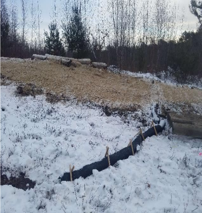
Fig 9: BMPs installed and straw broadcast on access road between Strs. 47-46. Viewing west. (01-06-20).
